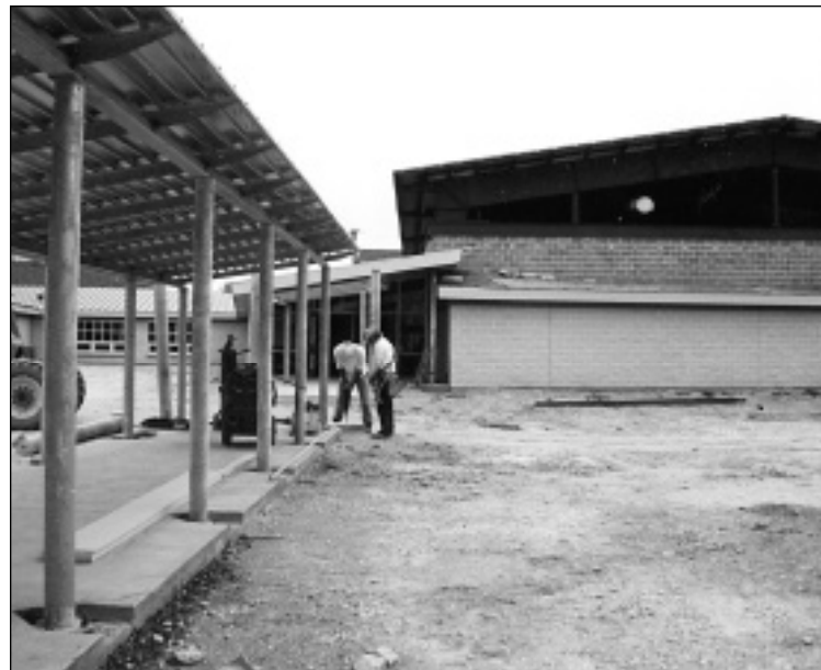
ON SCHEDULE — The almost-15,000 sq. ft. Indoor Recreation Center is being built with a Texas Parks and Wildlife Dept. matching grant.
